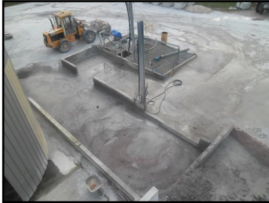
Plant sedimentation platform
