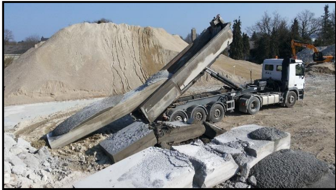
Detachment of a concrete block
